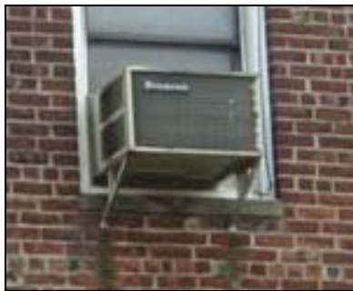
Figure 10: an AC unit that does not require a permit (LPC, 2007).
