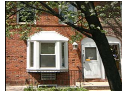
Figure 11: a flush-mounted AC unit beneath a bay window (LPC, 2007).
